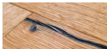
Partially filled cracks
